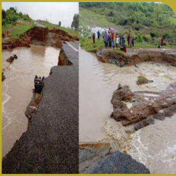
Infrastructures affected by floods (URT)
